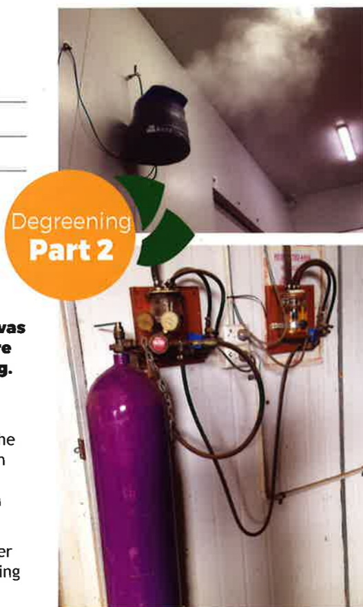
TOP: Generating high humidity in degreening rooms is essential.
